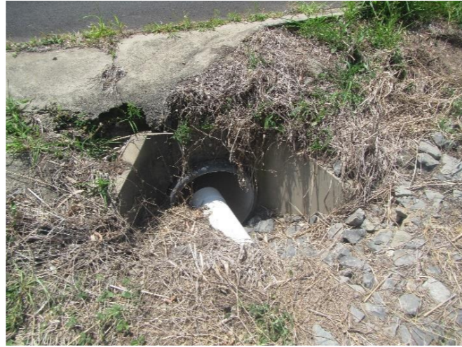
Plate 11: Stormwater diversion on southern side of Savage Street directing waters to northern side of Savage Street and into project site
